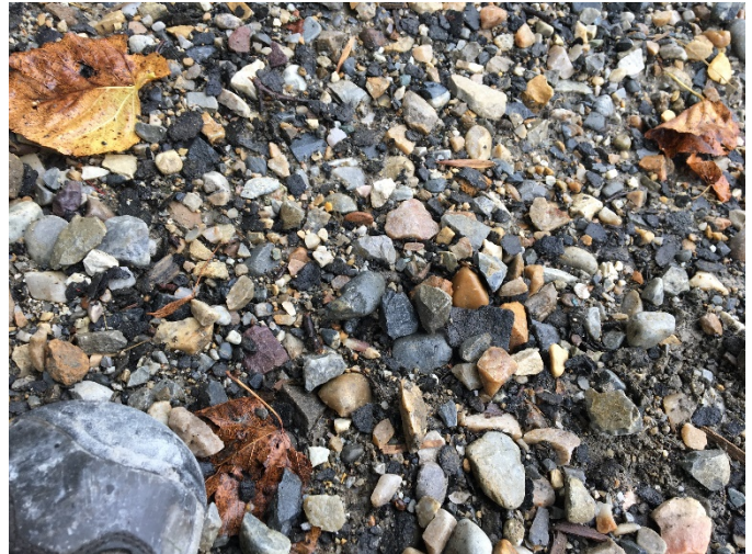
Loose Shoulder Material
