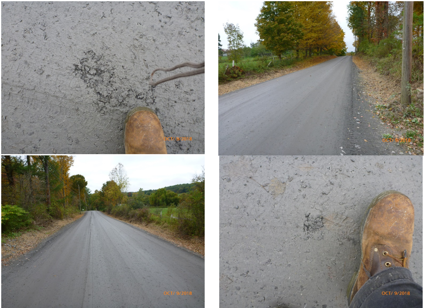
Figure 11: Shaftsbury post resurfacing condition
